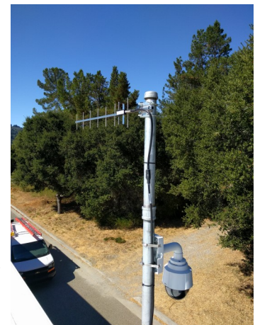
Video camera at remote site, used to monitor access
