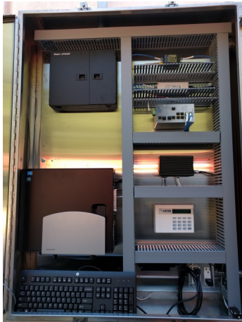
Remote panel approx. 700 ft away from main facility
